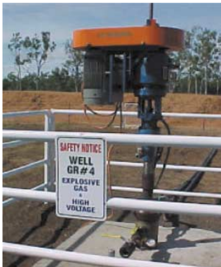
Figure 10b: Photograph showing a progressive cavity pump wellhead installation in Australia comparable to that being installed in the Dobson well.
