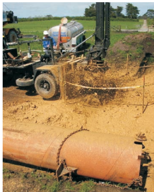
Fig 8. “Holes-R-Us” drilling the gun pit. The steel liner for the hole is in the foreground. Behind the truck mounted Auger unit is the tanker with spare mud.
