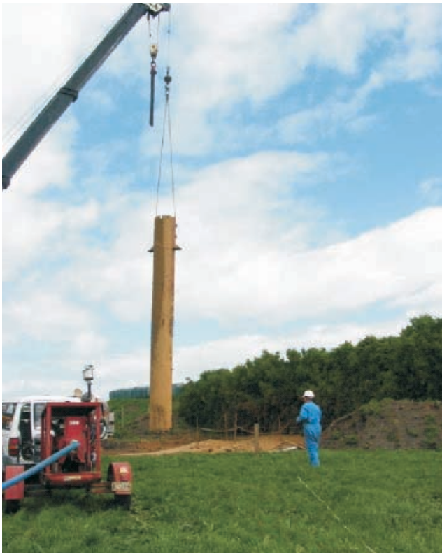
Fig 9. Lowering the Steel pipe into the gun pit. The spiral welded pipe is 9m x 0.91m x 10mm and weighs 2 ton.
