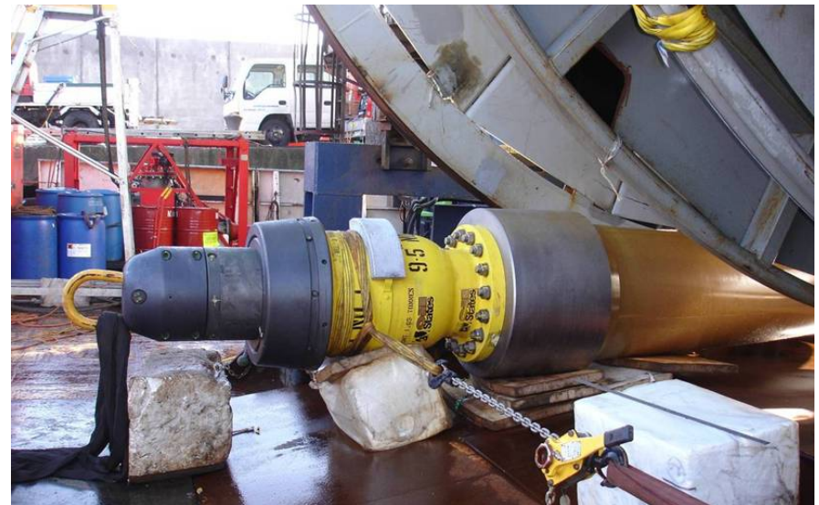
Riser pull-in assembly
